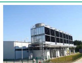
Cooling tower and heat transfer building
